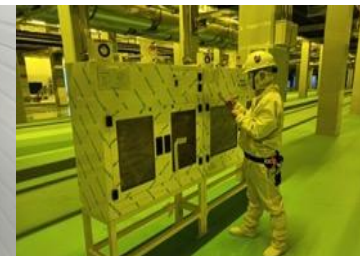
VMB阀箱材料验收 Acceptance of VMB valve box materials
