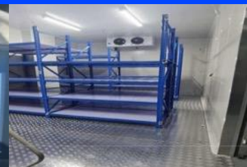
库房温湿度测试 Air volume testing
